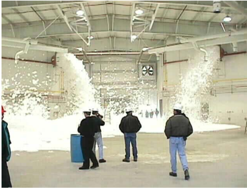
Figure A2.1. Low-Level High-Expansion Foam Wall-Mounted (Adjacent Leading Wing Edge) Generators' Initial Discharge
