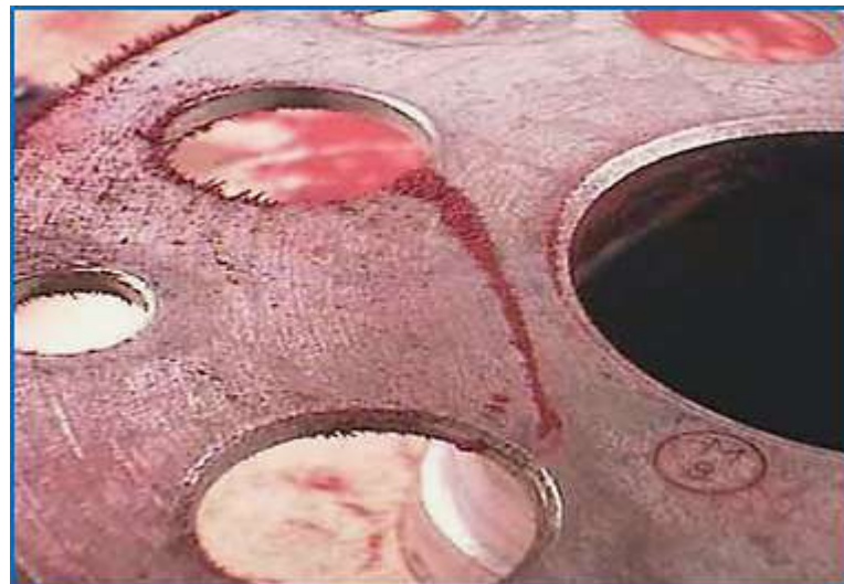
Indication of cracks originating at a fastener hole
