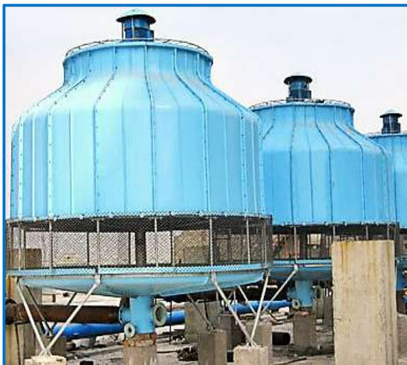
Mechanical Draft Towers
