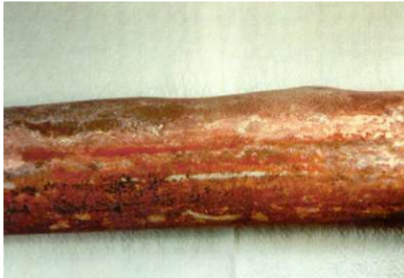
Figure 1.7 Metal Fatigue on Boiler Tube
