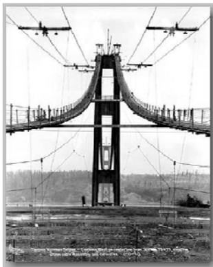
Tacoma Narrows Bridge Under Construction (University of Washington Libraries, Special Collections, PH Coll. 11.19)
